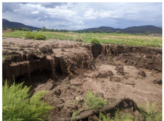
Severe Erosion Damage - Copeland Detention Facility
